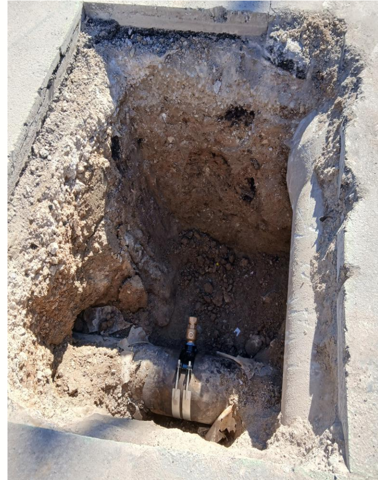
10"x1.5" saddle on DI water main
