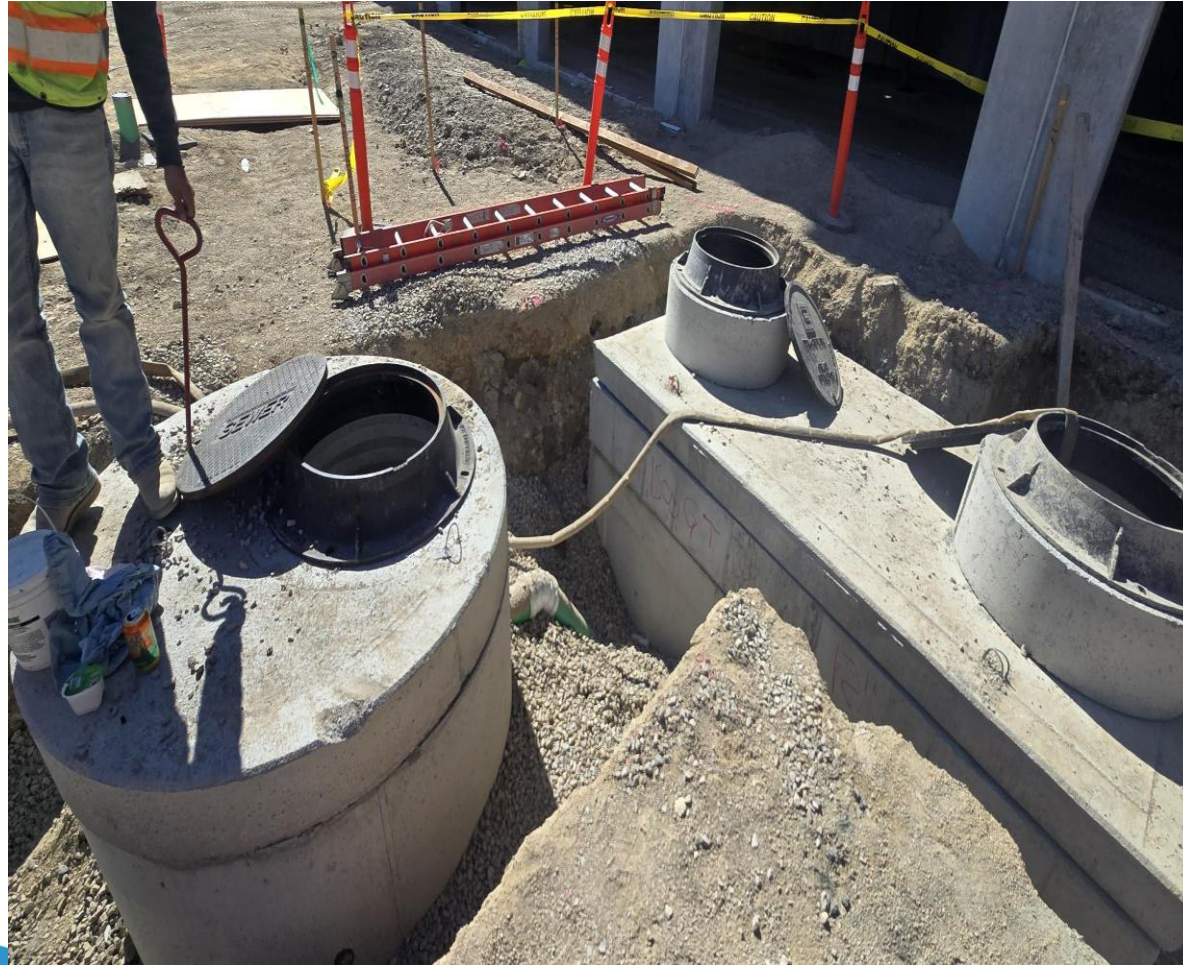
1,500-gallon grease interceptor and sample manhole
