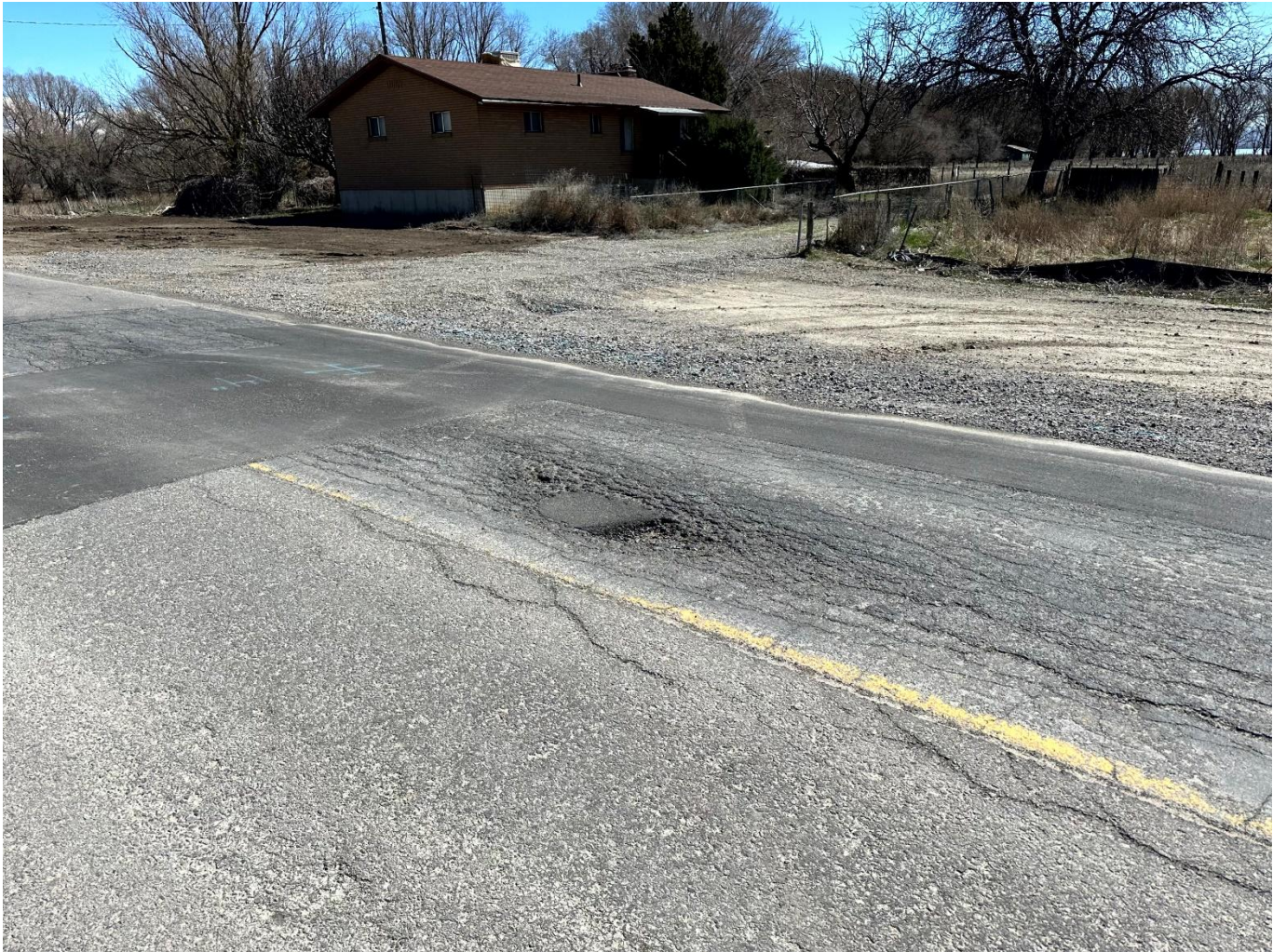
Figure 3. Typical Surface Condition of the Pavement (145 N)
