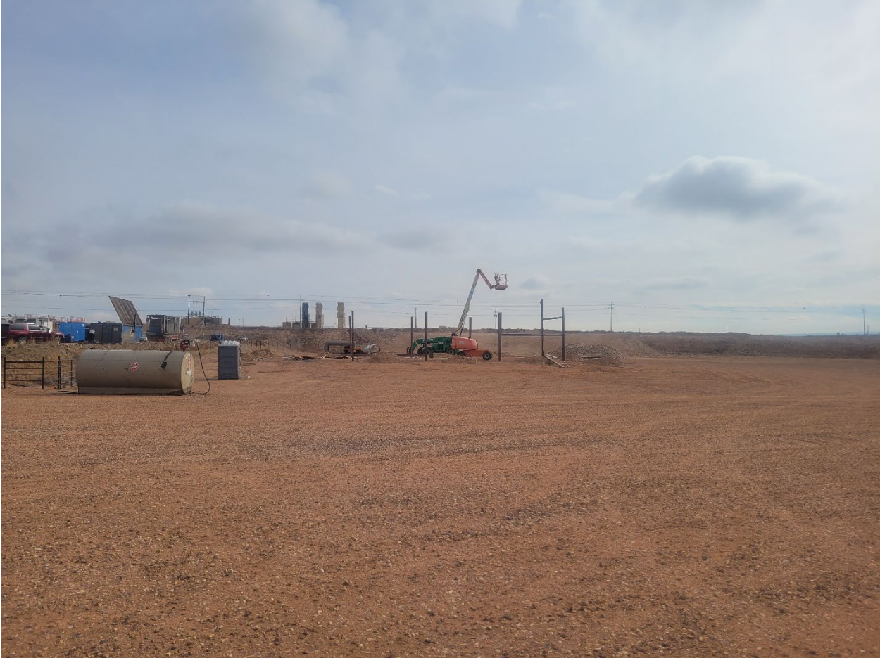
Picture 3: Footers for the building that will be moved from other location.
