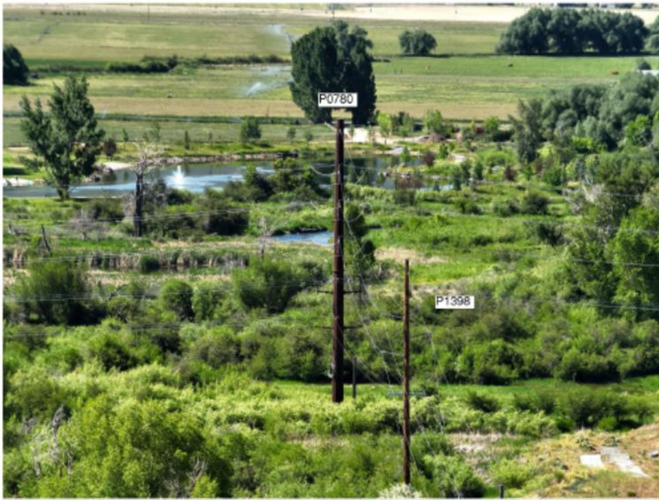
EXISTING POLE(S) - VIEW #1
