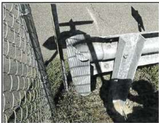
Railing 2 Distortion at South End
