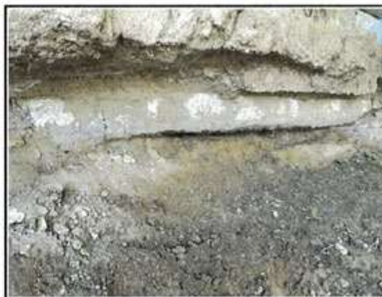
Abutment 1 Scour With Up to 20 IN Undermining
