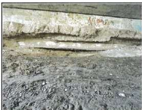
Abutment 1 Scour With Up to 20 IN Undermining
