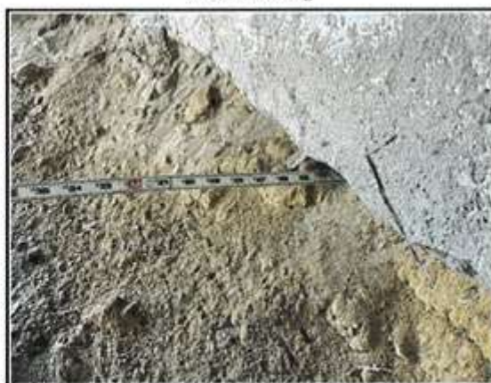
Abutment 1 Up to 24 IN Undermining
