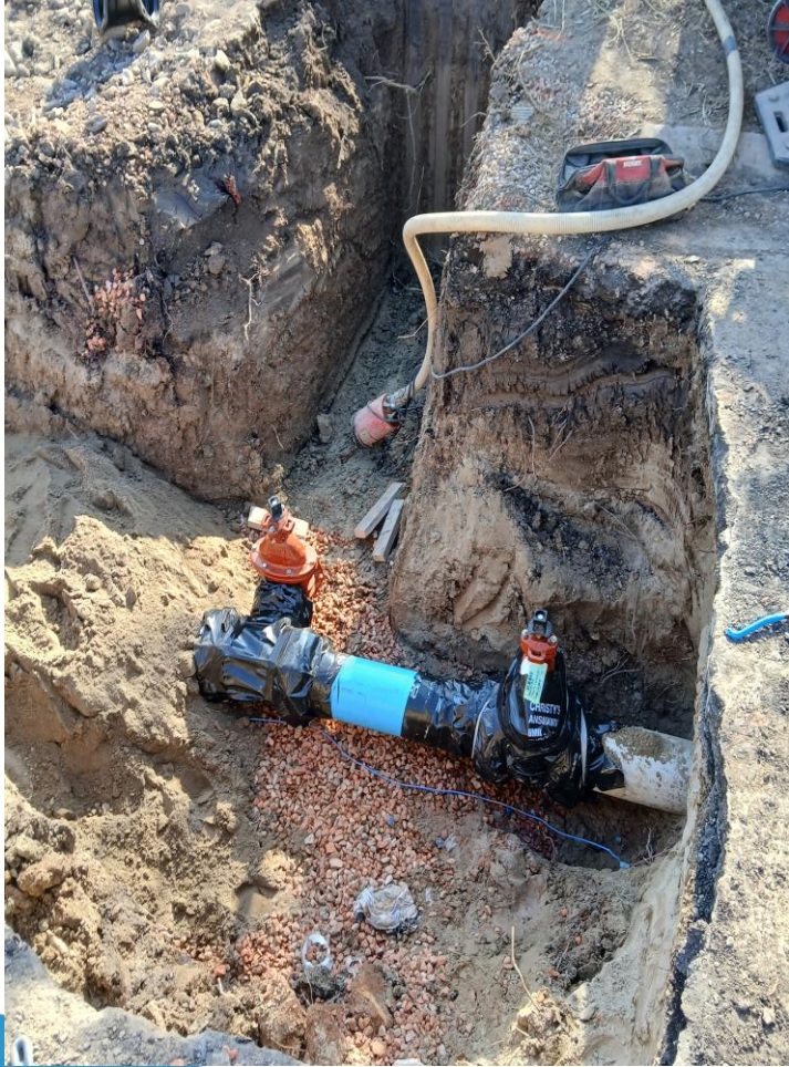
8" water line with inline & hydrant valve
