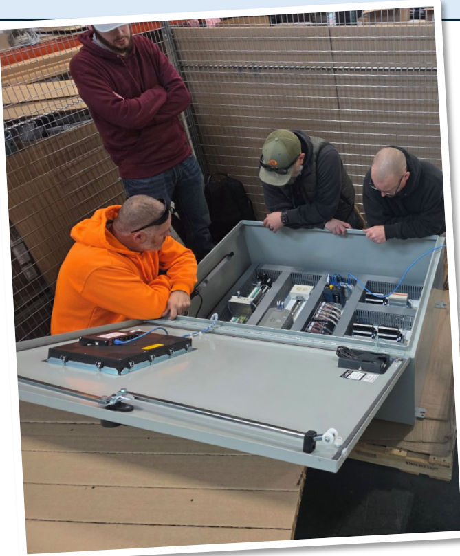
Operators testing the new panel for Anderson Treatment Plant.
