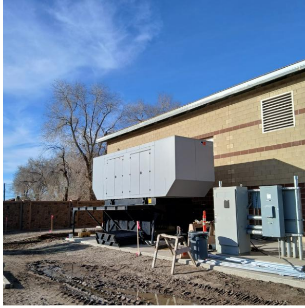
Anderson WTP – Generator installed
