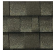
Roof Weathered Wood
