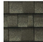
Roof Weathered Wood
