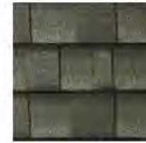
Roof Weathered Wood
