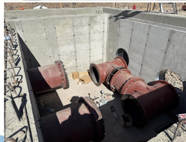
24" Piping and Valve Vault on Northeast Side of Anderson WTP
