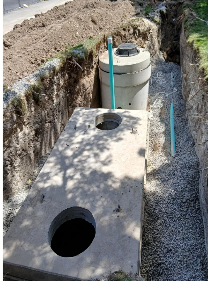
1,500-gallon grease interceptor with sampling manhole
