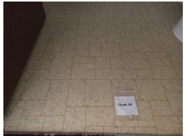
Photo #64 HA64: Tan rectangle and square pattern vinyl sheet flooring and mastic, asbestos containing
