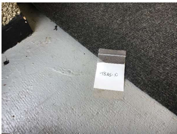
Photo #47 HA47: Remnant carpet mastic, asbestos containing
