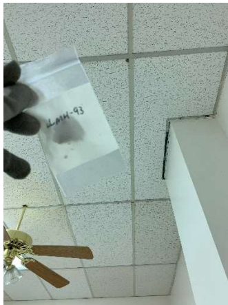
Photo #33 HA32: White 2'x4' ceiling tile with long gouges, not asbestos containing
