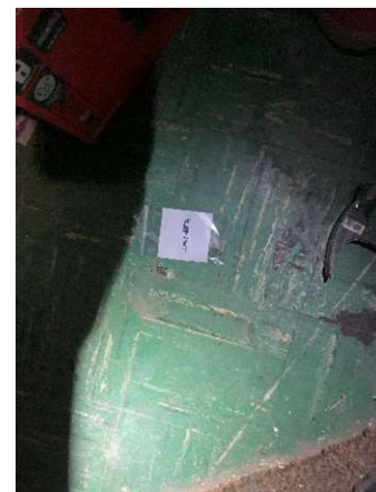
Photo #24 HA23: Green 9"x9" floor tile with white streaks and mastic, asbestos containing
