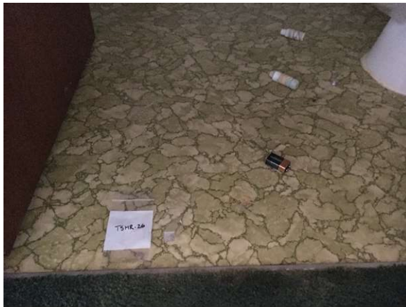
Photo #63 HA63: Green stone floor pattern vinyl sheet flooring and mastic, asbestos containing
