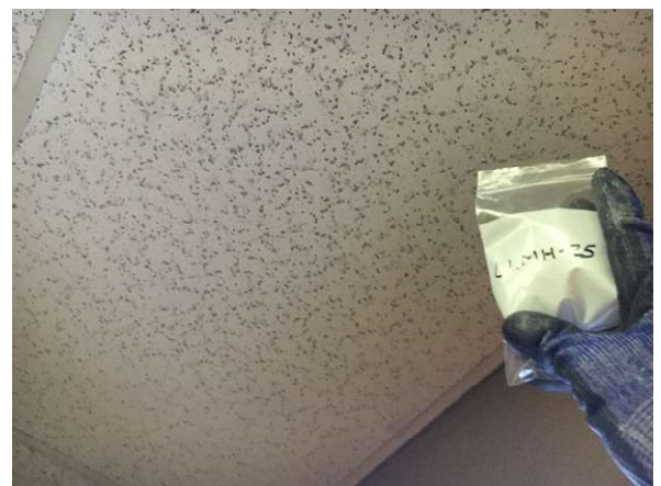
Photo #6 HA5: White 2'x4' ceiling tile with many small gouges and pinholes, not asbestos containing
