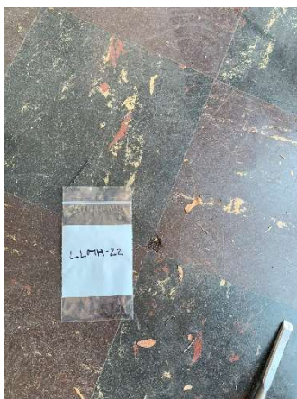
Photo #5 HA4: Dark red 9"x9" floor tile with white and red streaks and mastic, asbestos containing
