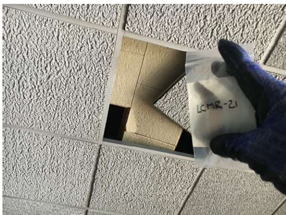
Photo #41 HA40: White 1'x1' "wall texture" pattern ceiling tile, not asbestos containing
