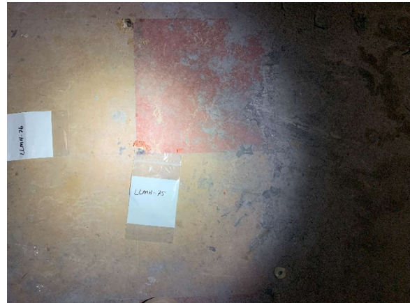
Photo #26 HA25: Red 9"x9" floor tile and mastic, asbestos containing
