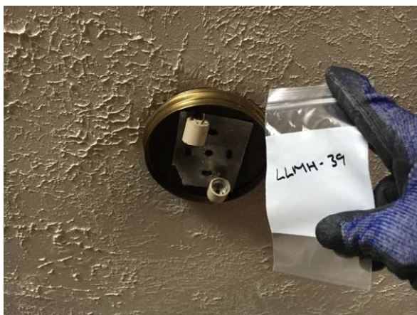
Photo #11 HA10: Heat shield (lamp fixtures), asbestos containing
