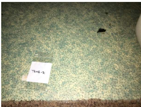
Photo #65 HA65: Blue and white small oblong shaped pattern vinyl sheet flooring and mastic, asbestos containing
