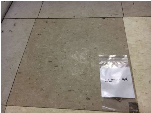
Photo #13 HA12: Brown 12"x12" floor tile and mastic and cementitious material, asbestos containing
