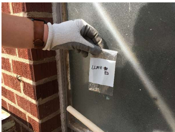
Photo #29 HA28: White window glazing, asbestos containing
