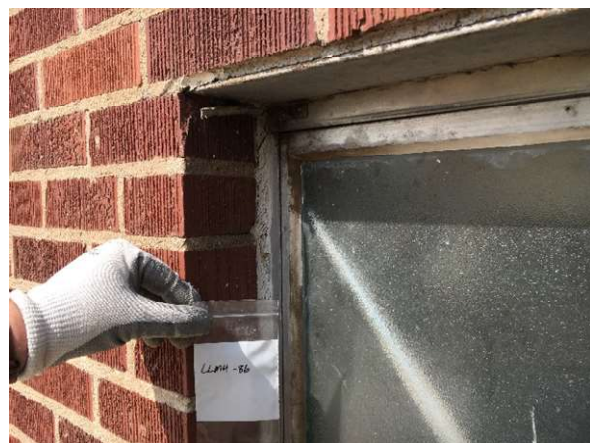
Photo #30 HA29: Beige window caulking, asbestos containing
