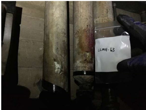
Photo #21 HA20: Corrugated pipe insulation, asbestos containing
