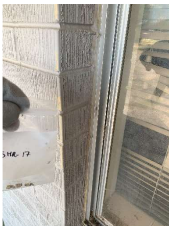
Photo #53 HA53: Window/door caulking, asbestos containing
