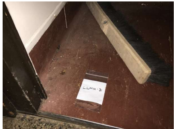
Photo #8 HA7: Red vinyl sheet flooring with white streaks and mastic, not asbestos containing
