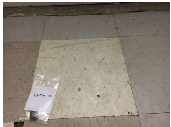
Photo #12 HA11: White 12"x12" floor tile and mastic and cementitious material, asbestos containing
