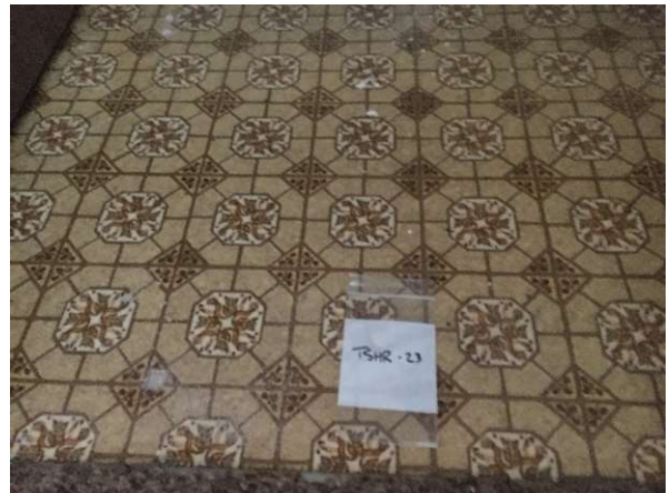
Photo #62 HA62: Yellowish brown flower pattern vinyl sheet flooring and mastic, not asbestos containing
