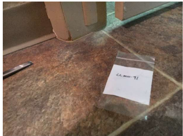
Photo #32 HA31: Brown flagstone pattern vinyl sheet flooring and yellow mastic (multiple layers), asbestos containing
