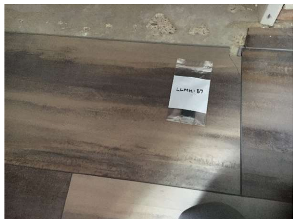
Photo #18 HA17: Wood pattern brown 12"x24" floor tile and mastic, not asbestos containing
