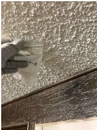
Photo #3 HA2: White popcorn ceiling texture, asbestos containing
