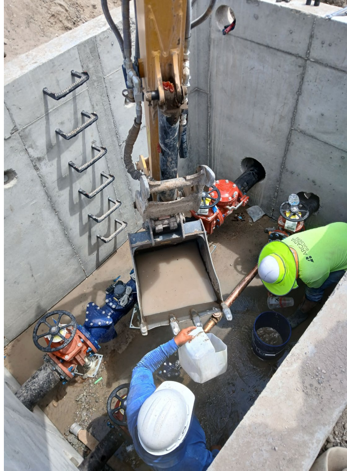
Plumbing 6" water meter vault
