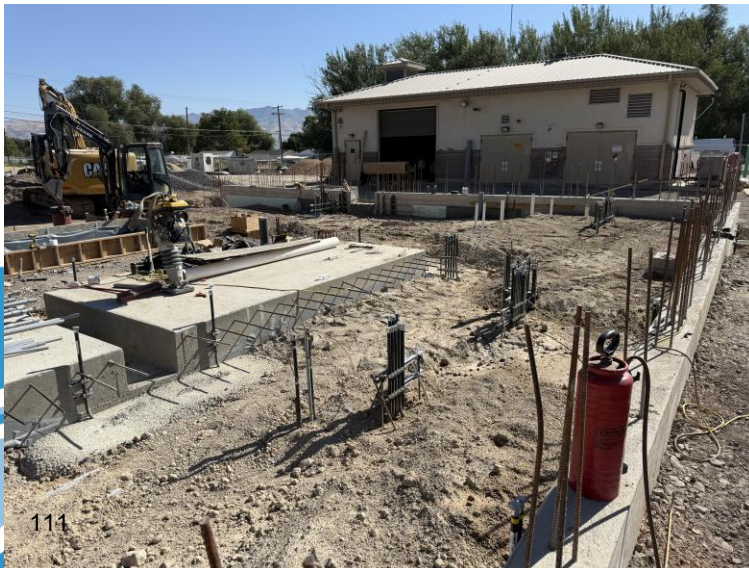
Electrical Conduit and Plumbing in Anderson WTP
