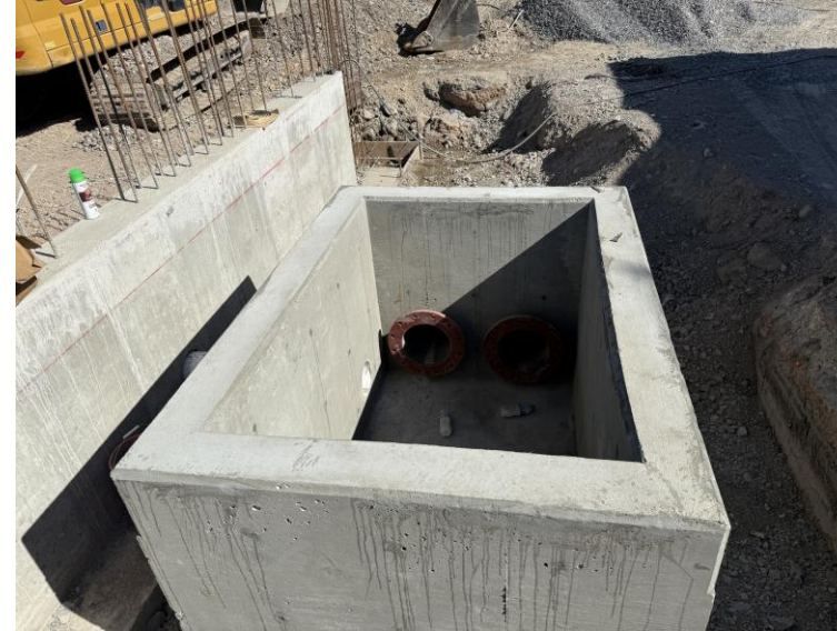
Pressure Filter Backwash Catch Basin on the Exterior East Side of Anderson WTP
