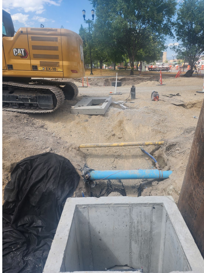
2" water lateral taps on 8" water main
