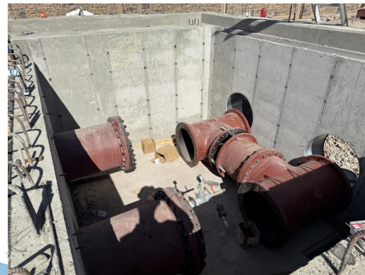
24" Piping and Valve Vault on Northeast Side of Anderson WTP
