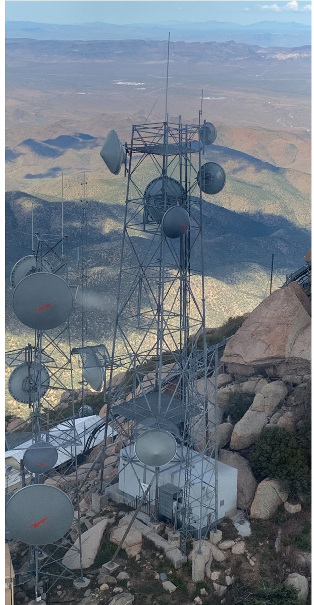
WAPA's transmission system operations depend on microwave radio installations like this communications site near Kingman, Arizona.
