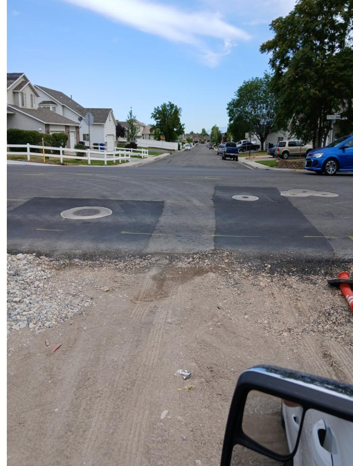
Manhole and water valve collars
