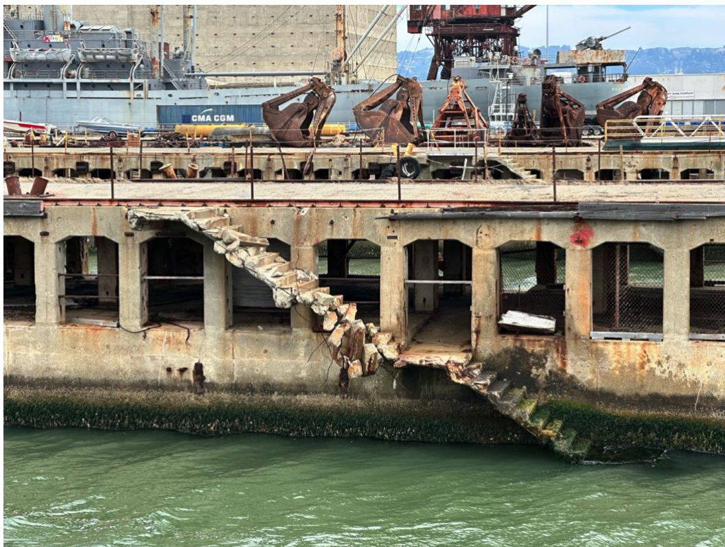
Example of physically deteriorating infrastructure at the Port.
