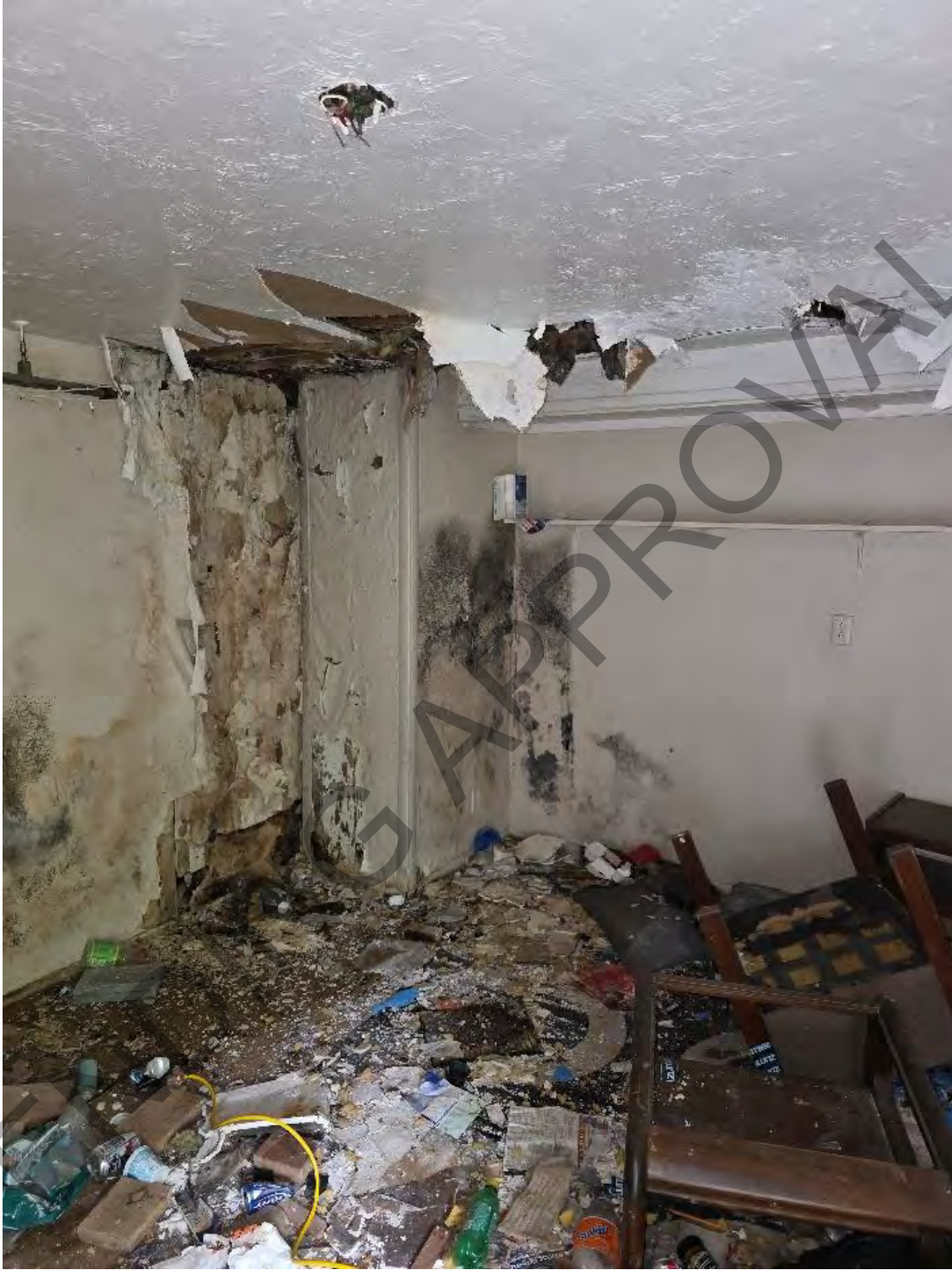
South Basement Apartment Living Room – Three (3) dead raccoons, feces, visible mold on all walls within the basement area.
