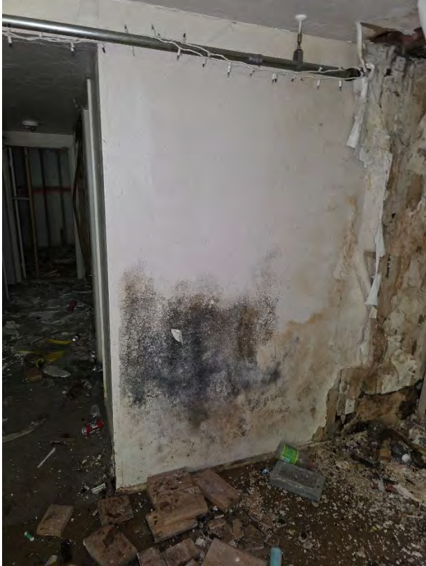
Basement South Apartment visible mold growth, animal feces and garbage
