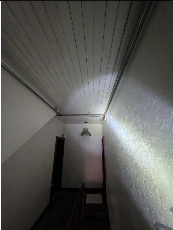
Green wood ceiling positive for lead
