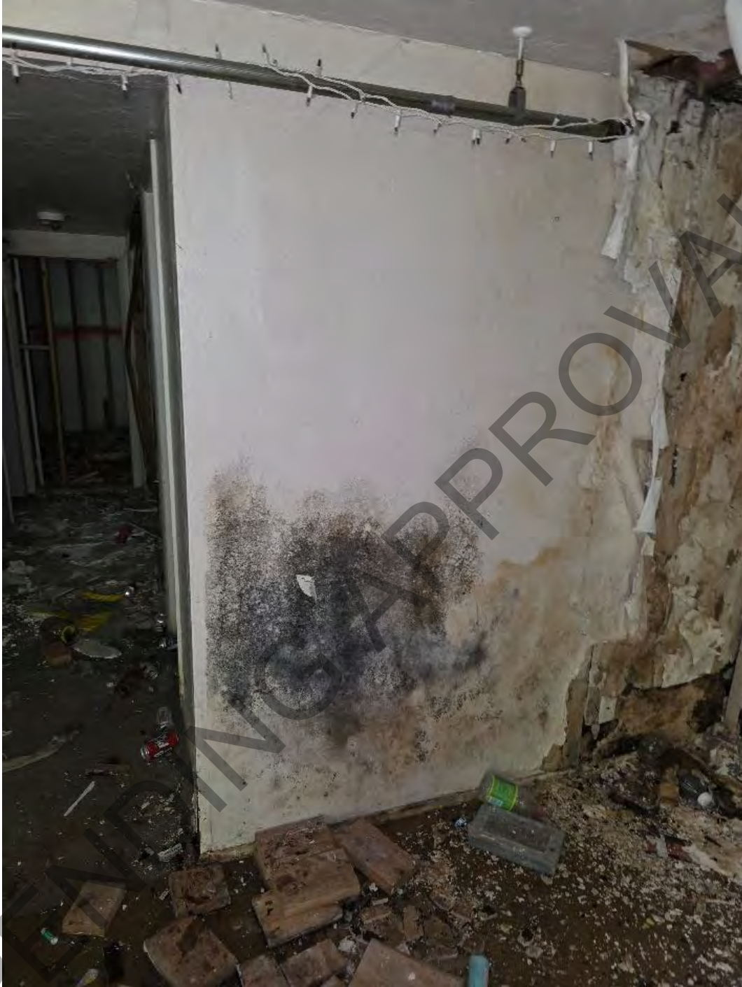
Visible mold growth on wood paneling Office 103/104.
