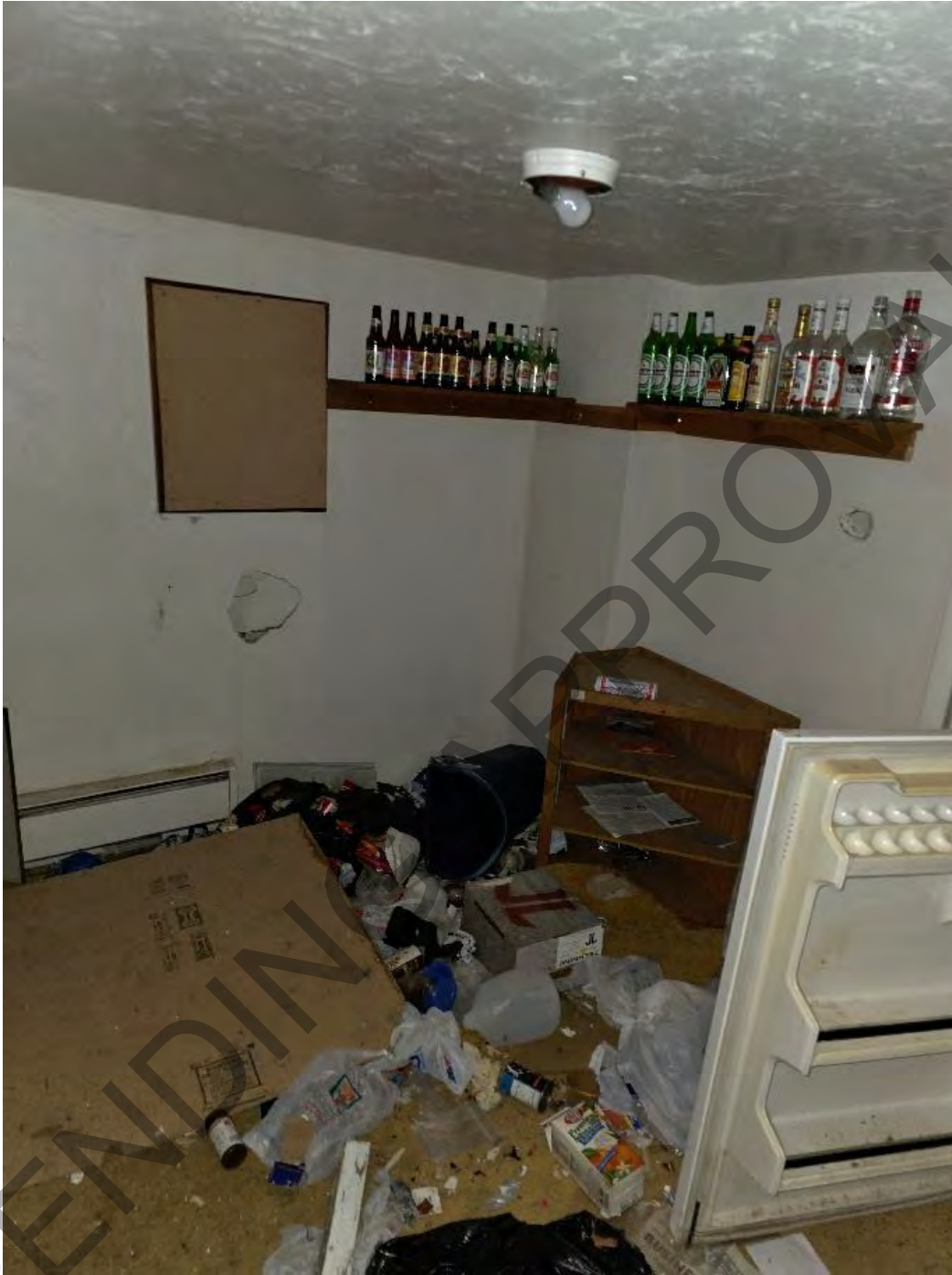
Basement South Apartment Kitchen with visible mold growth and feces.
