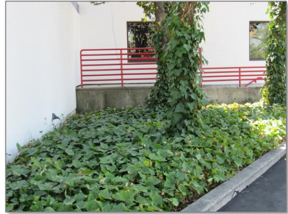
Figure 7: Downspout disconnected from parking lot
