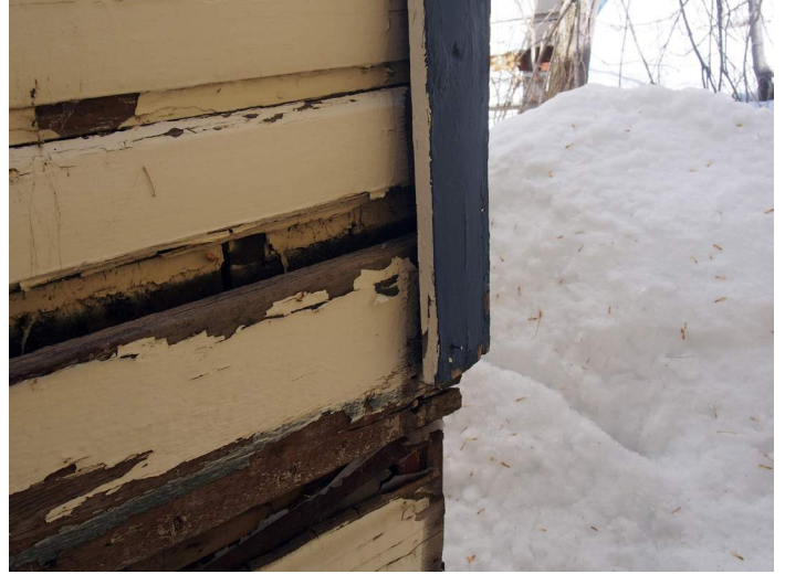
South facade siding and trim fail - opposite
