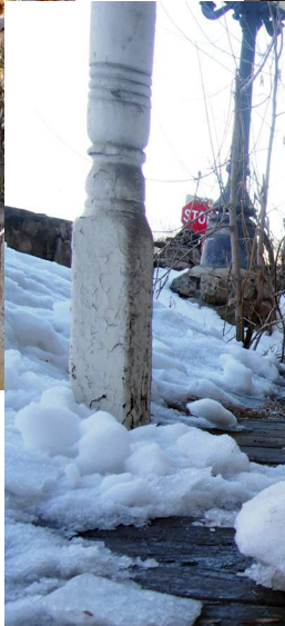
Base of Front Porch Post
