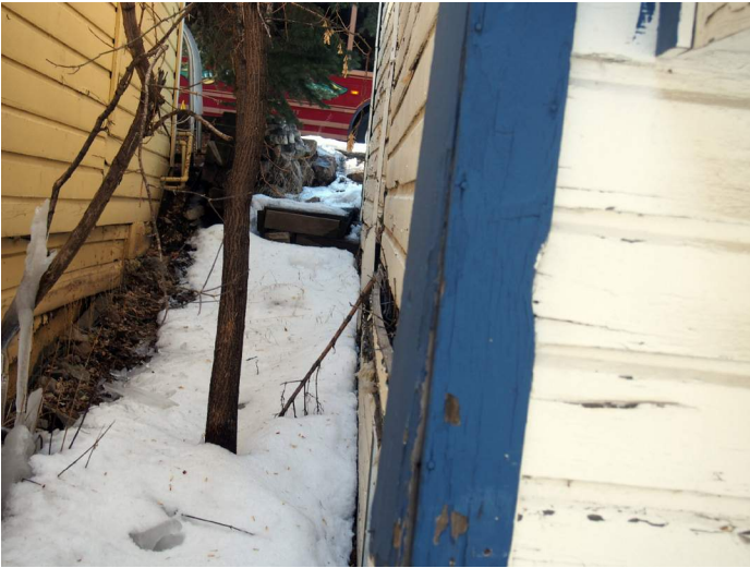
Bowing South wall
