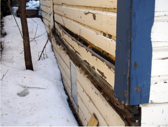
South facade siding and trim failing
