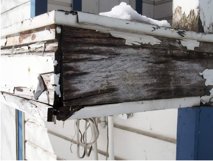
Trim compromised at rear Level 1 deck
