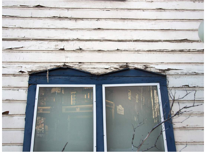
Missing finials on window trim and peeling paint
