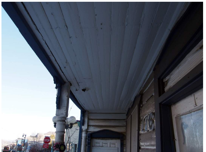
Front Deck soffit bowing
