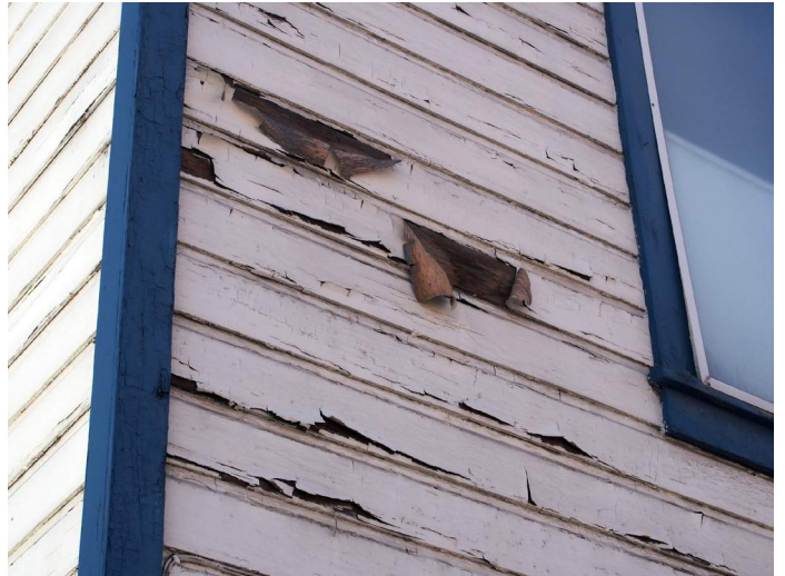
Example of Peeling paint on West Facade
