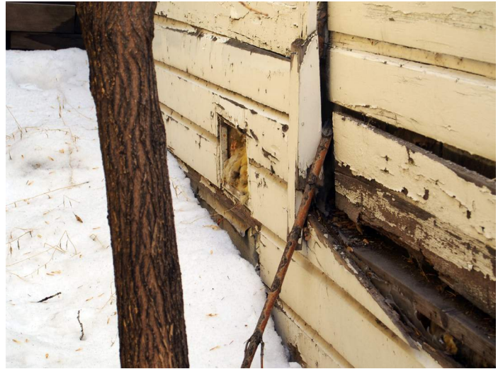
South facade trim issues
