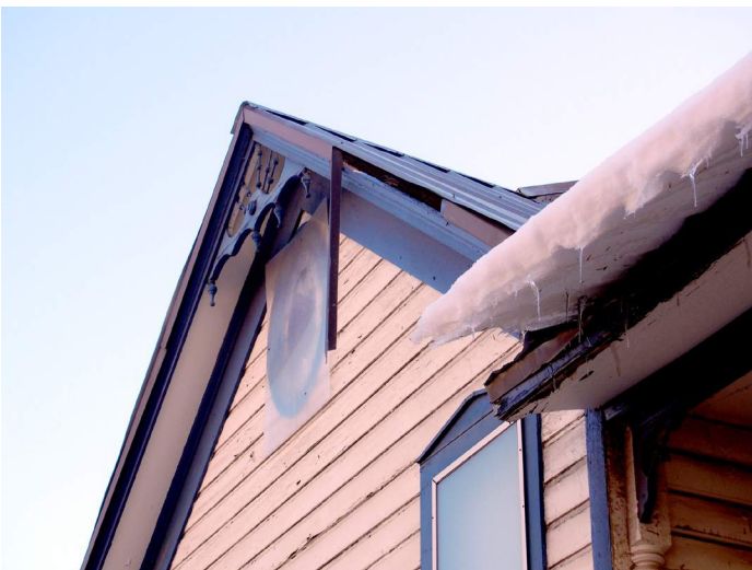
Drip edge failing and saturated soffit
