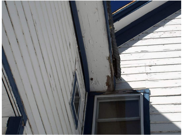
East gabled section soffit compromised
