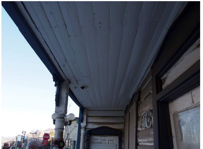
Front Deck soffit bowing
