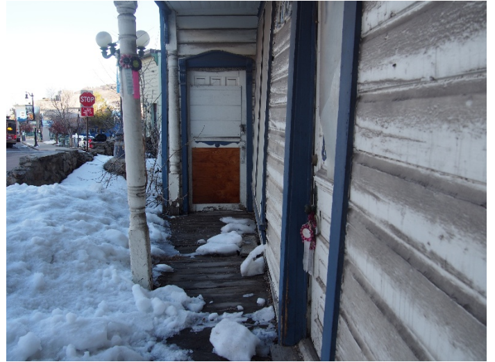
Figure 5- Main St. Buckling Wall
