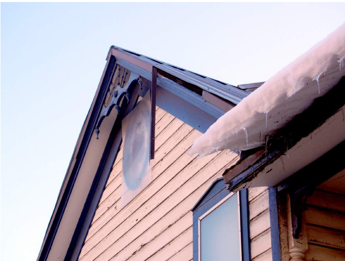
Drip edge failing and saturated soffit
