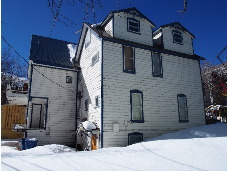
Figure 1- NE Corner (structure leaning)
