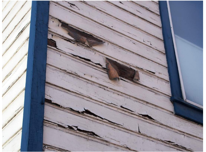
Example of Peeling paint on West Facade
