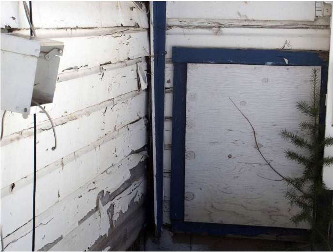
Peeling trim and paint at South and East inside corner
