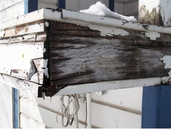
Trim compromised at rear Level 1 deck
