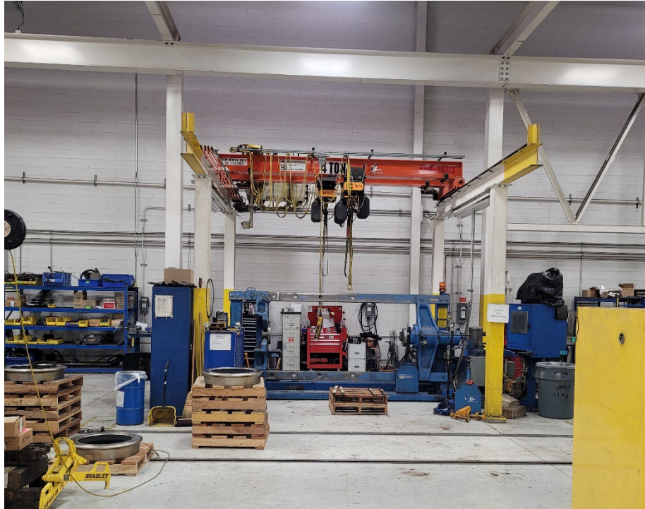
Figure 2 - Existing JRRSC Wheel Press
