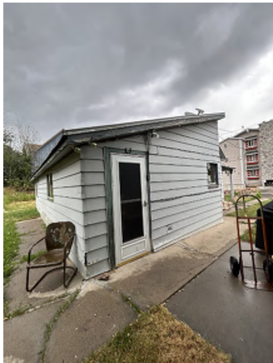
Rear addition with no perimeter band
