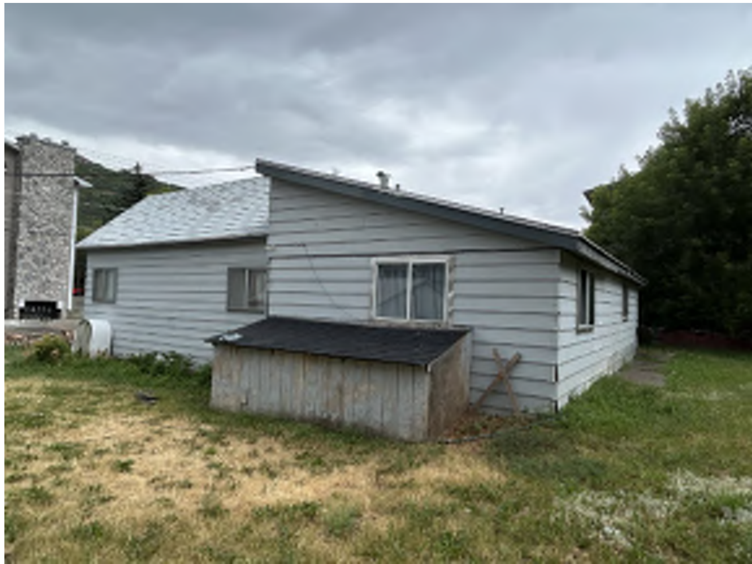
Rear addition with no perimeter band
