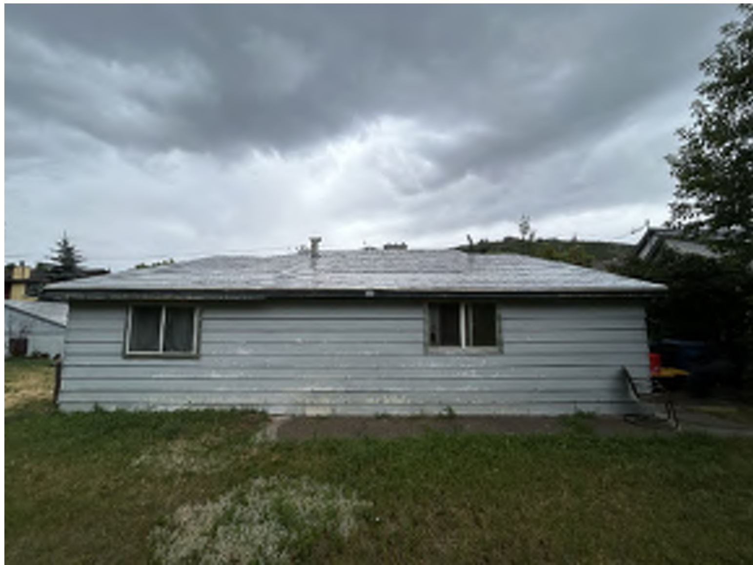
Rear addition with no perimeter band
