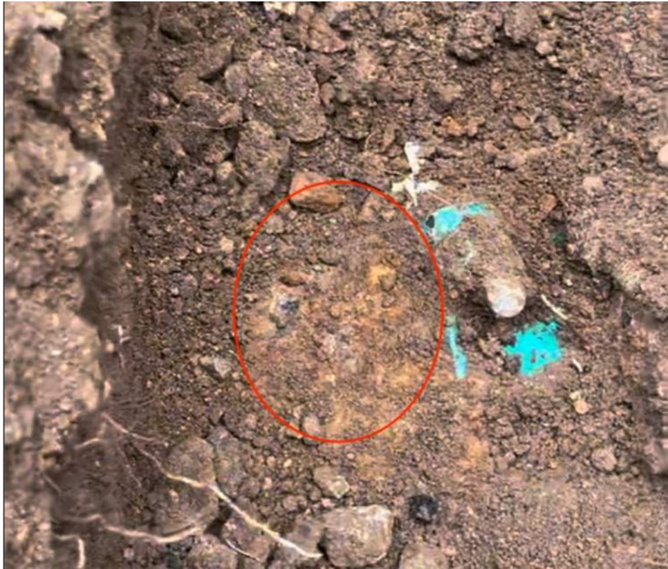
Corrosion on top of main service line – 329 Bern Way
