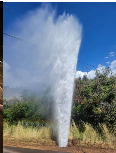
St. Moritz Water line break – 9/15/24
