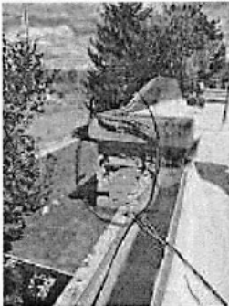
Activity Center Brick Damage - 2.jpeg 596K
