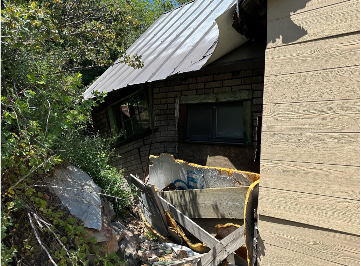
Figure 6: Looking northerly, the rear of Addition C clad in faux brick panels, showing damage, which will require extensive bracing to lift.
