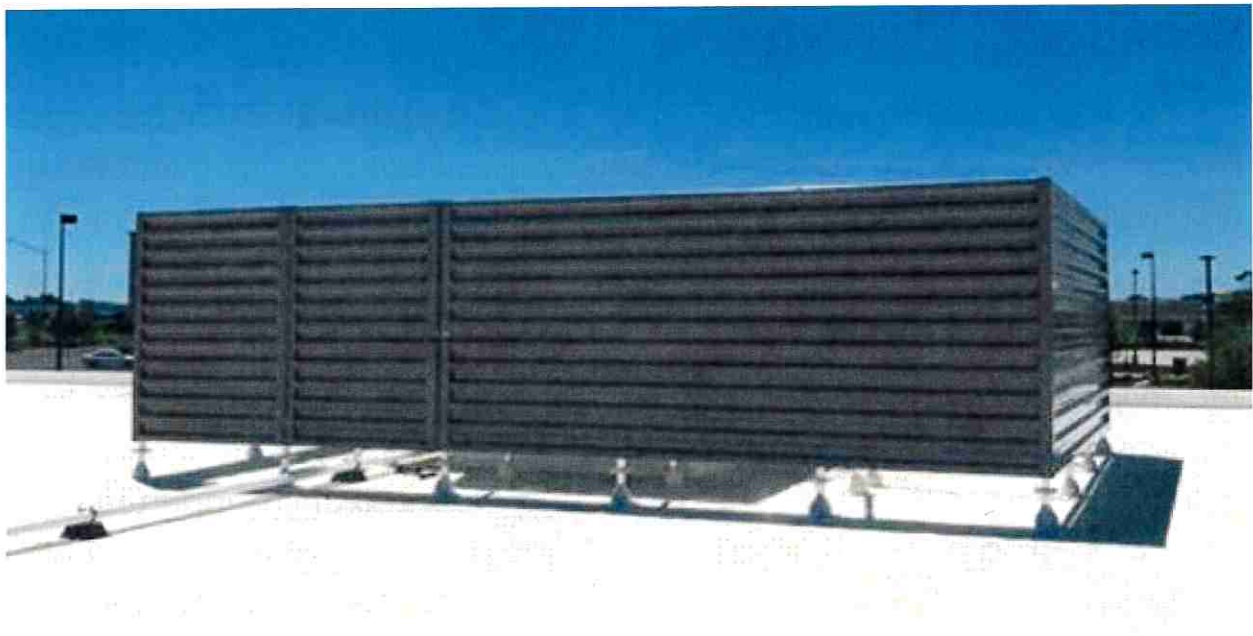
Roof top equipment screening. Photo credit to Roofline.
