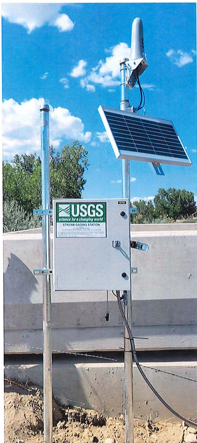
Figure 1. Gage shelter with data logger, solar panel, 12v battery and telemetry antenna. Example location: Ashley Creek near Jensen, UT
