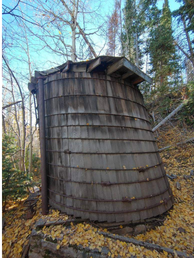
Photo 2—Water tank looking East
