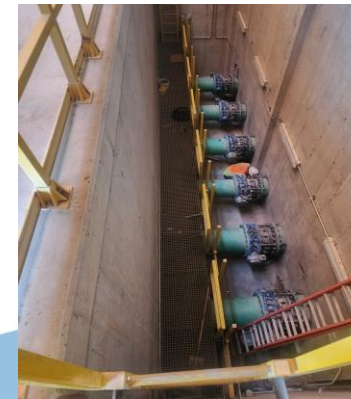
Pump suction piping
