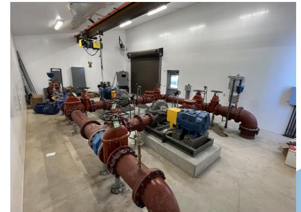
Booster Pump Station
