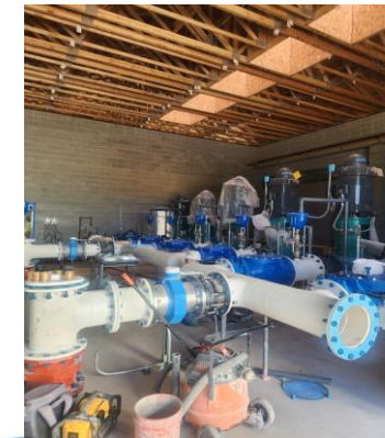
Pump motors and discharge piping
