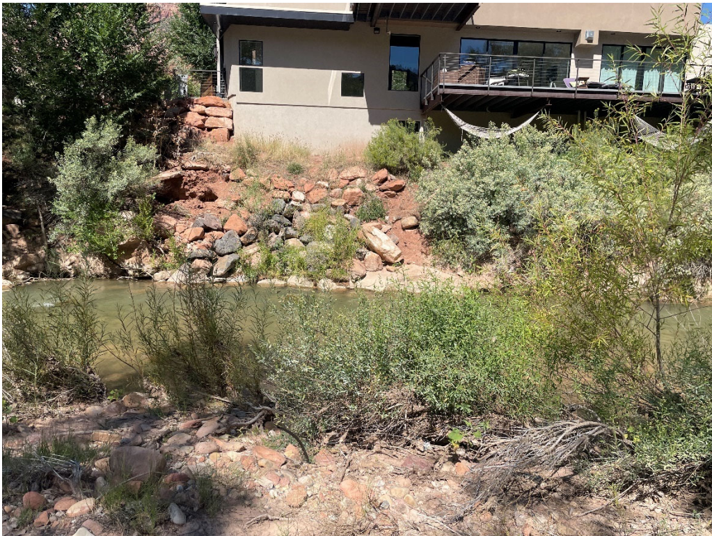
Figure 5 – September 26, 2023. Looking across the North Fork of the Virgin River from the left (east) overbank at the existing erosion protection, located adjacent to the downstream residence. This erosion protection has previously been damaged by high flow events.
