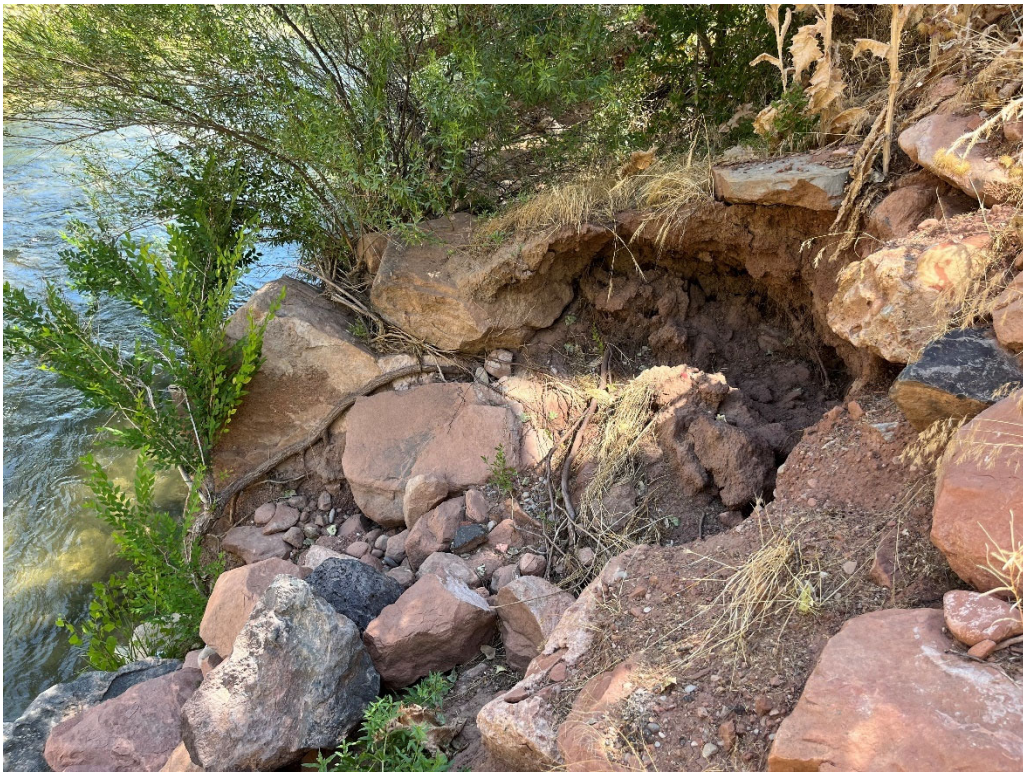
Figure 6 – September 26, 2023. Closeup image of the damaged existing erosion protection adjacent to the downstream residence.
