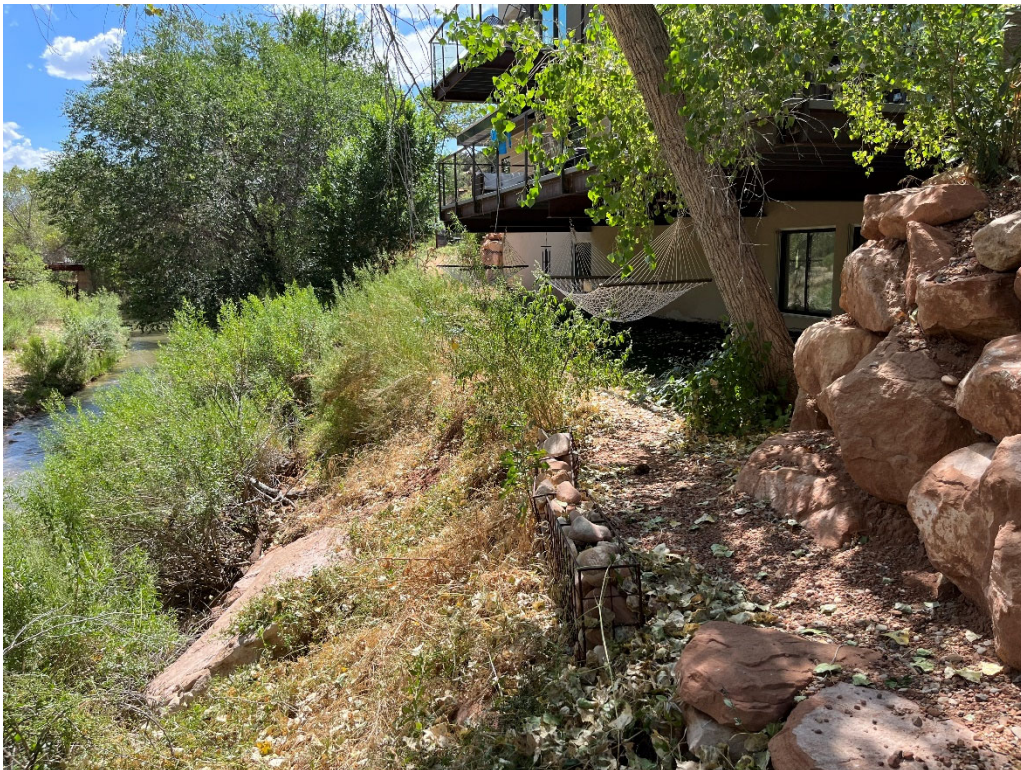
Figure 9 – July 27, 2023. Looking downstream along the right (west) overbank adjacent to the retaining wall. This image depicts the proximity of the residential infrastructure to the top of the bank. A narrow band of riparian vegetation is present at the base of the bank.
