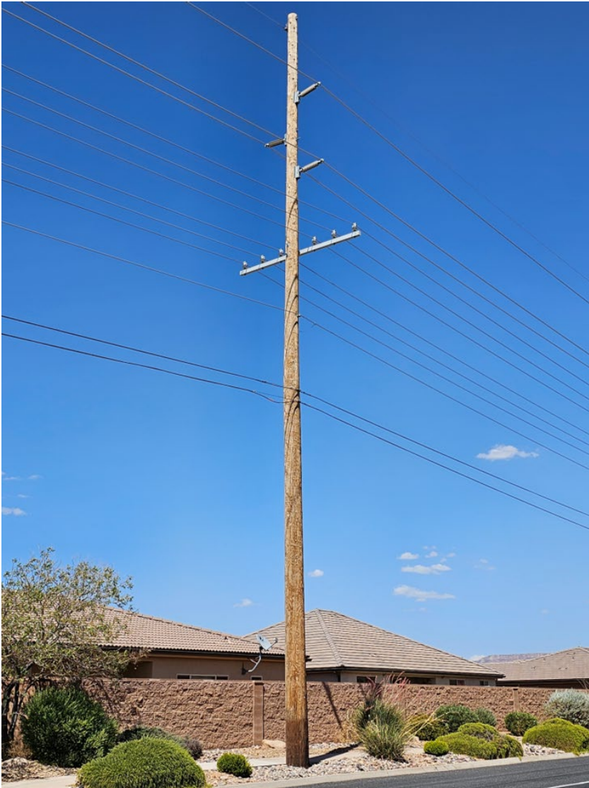
Structure E. Static wire (lightning protection and sometimes contains fiber optics inside it) at the top. Single circuit of transmission lines and double circuit of distribution lines underbuild with phone and cable under the distribution. Wood pole. Approx. 65' high.
