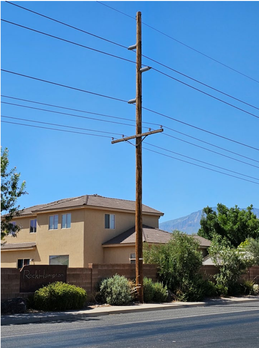
Structure D. Static wire (lightning protection and sometimes contains fiber optics inside it) at the top. Single circuit of transmission lines and single circuit of distribution lines underbuild. Wood pole. Approx. 52' high.
