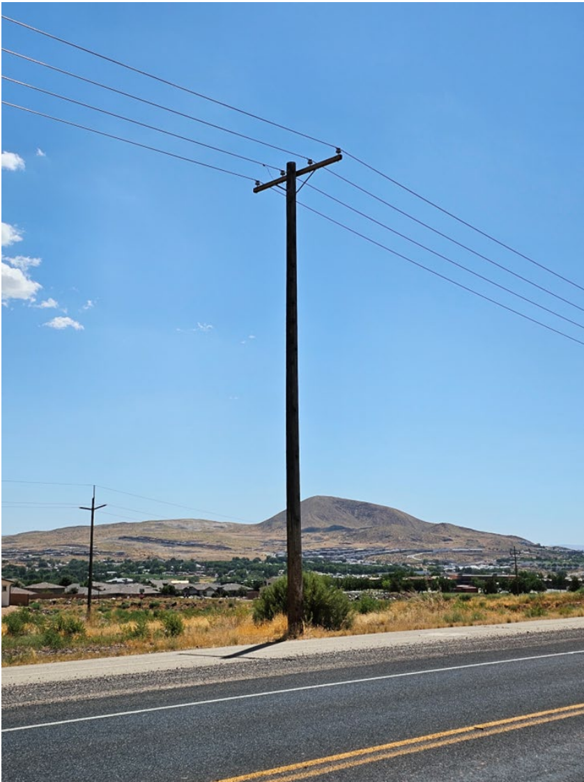
Structure A. Single circuit of distribution lines. Wood pole. Approx. 38' high. (In the background is a 69,000 Volt transmission pole.)
