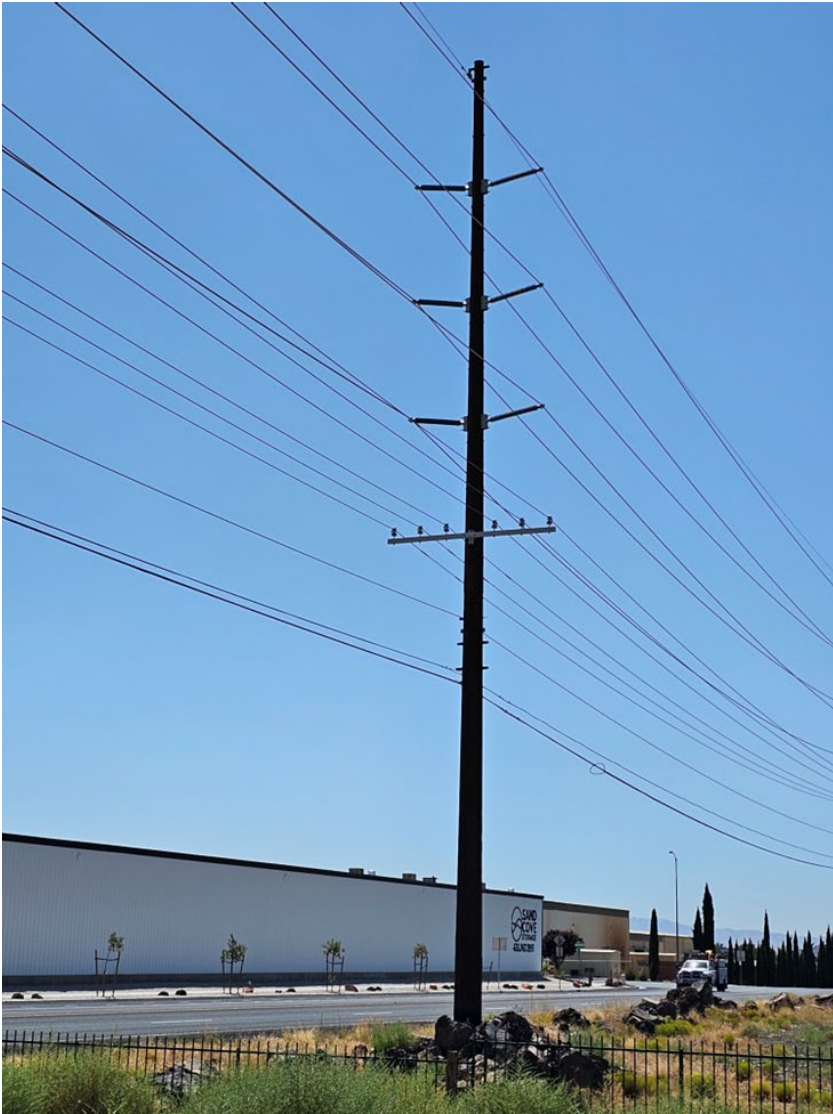
Structure F. Static wire (lightning protection and sometimes contains fiber optics inside it) at the top. Double circuit of transmission lines. Double circuit of distribution lines underbuild with phone and cable under the distribution. Steel poles. Approx. 79' high.
