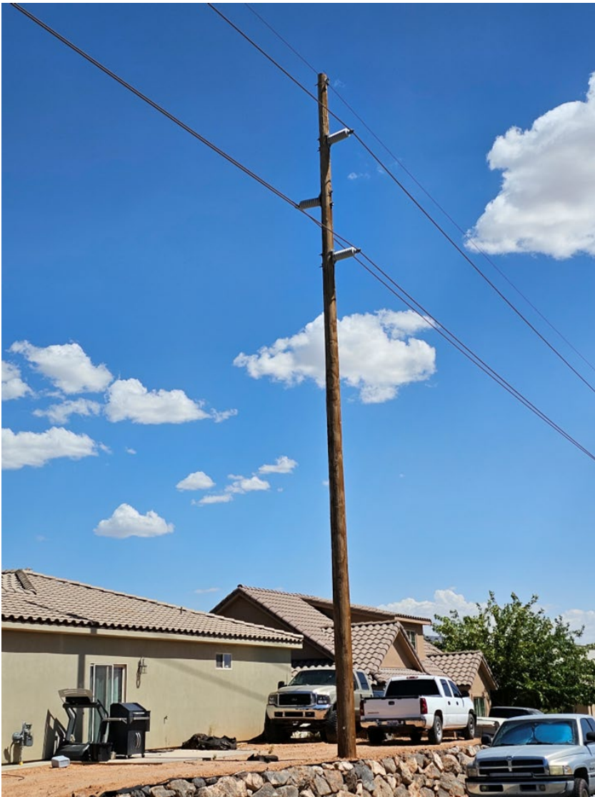
Structure C. Static wire (lightning protection and sometimes contains fiber optics inside it) at the top. Single Circuit of transmission lines. Wood pole. Approx. 52' high.
