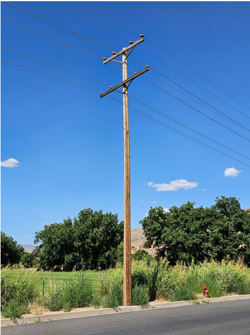
Structure B. Double circuit of distribution lines. Wood pole. Approx. 43' high.
