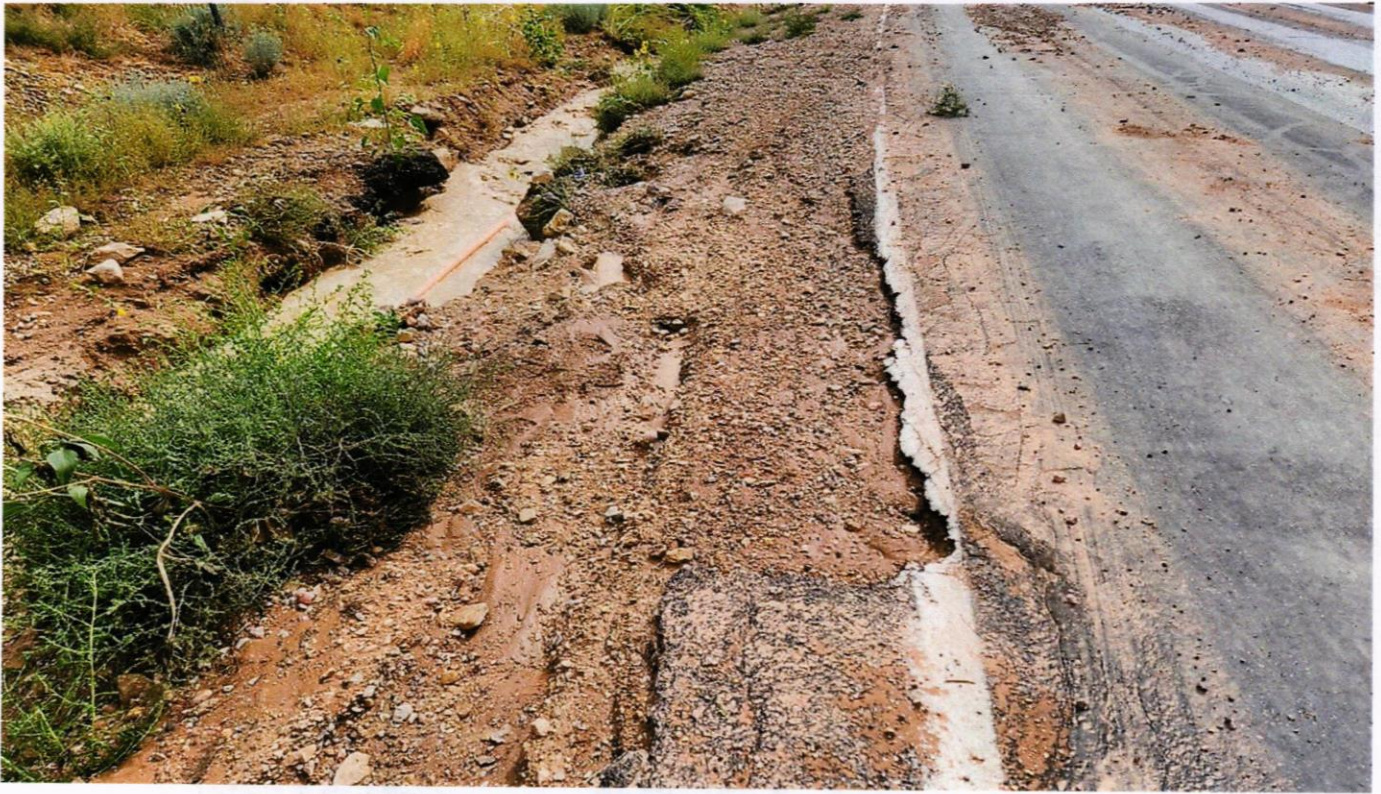
Road damage and gas lines exposed as a result of delayed shoulder, curb and gutter installation.
