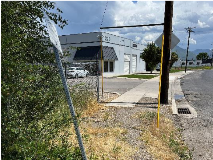
*Missing sidewalk segment along Central Avenue at UP underpass
