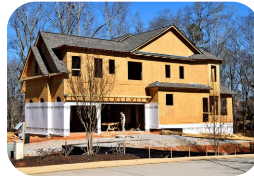
Cost to replace or construct a similar property
