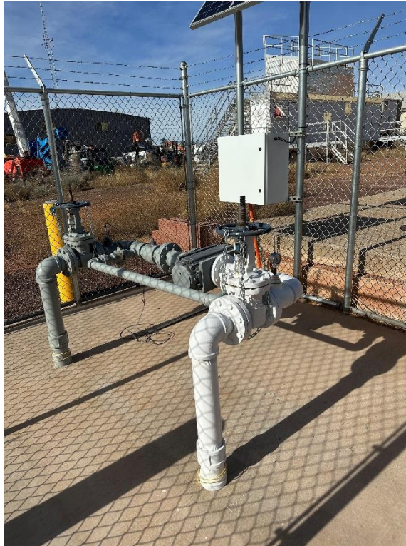
(Colorado City Natural Gas Gate Station)
